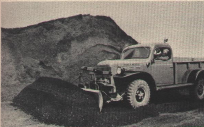
Spreading fill. Plenty of power for the toughest jobs . . . with efficient, economical operation.
