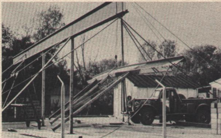
Erecting steel. Front end winch raises steel building sections easily and conveniently.
