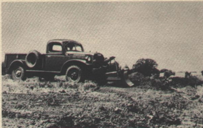
Grading and filling . . . with loose earth . . . is another Power-Wagon operation in which 4-wheel traction is important.
