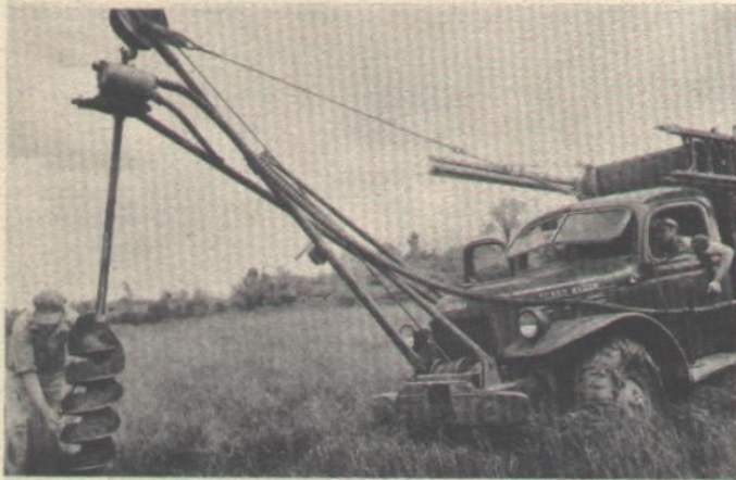
Hole drilling. Front end mounted drill expedites pole hole drilling in out-of-the-way places. Operator has clear vision from cab.
