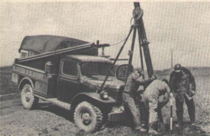
Pole placement. Utilizing drill tripod and power winch, poles are raised and placed in pole holes.
